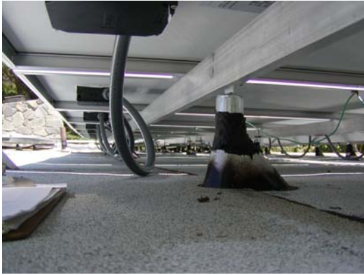
Figure 5 (incorrect) Flex exposed to physical damage
